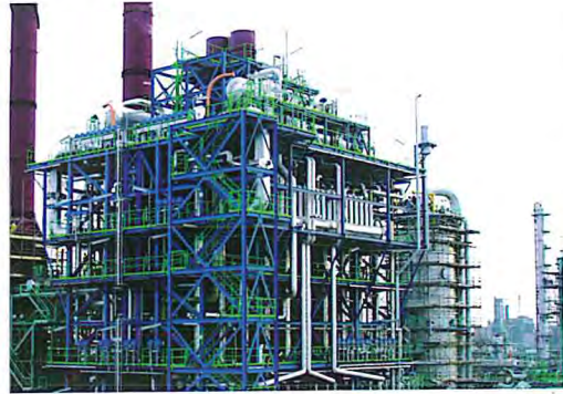
Transfer-line exchanger in an ethylene cracker.
