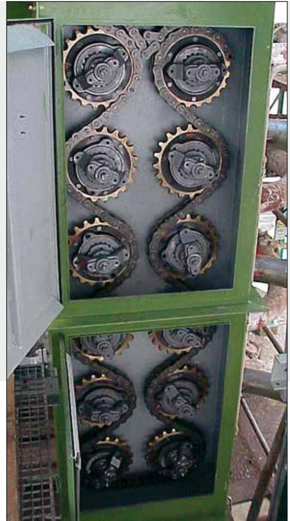
Replacement drive system
