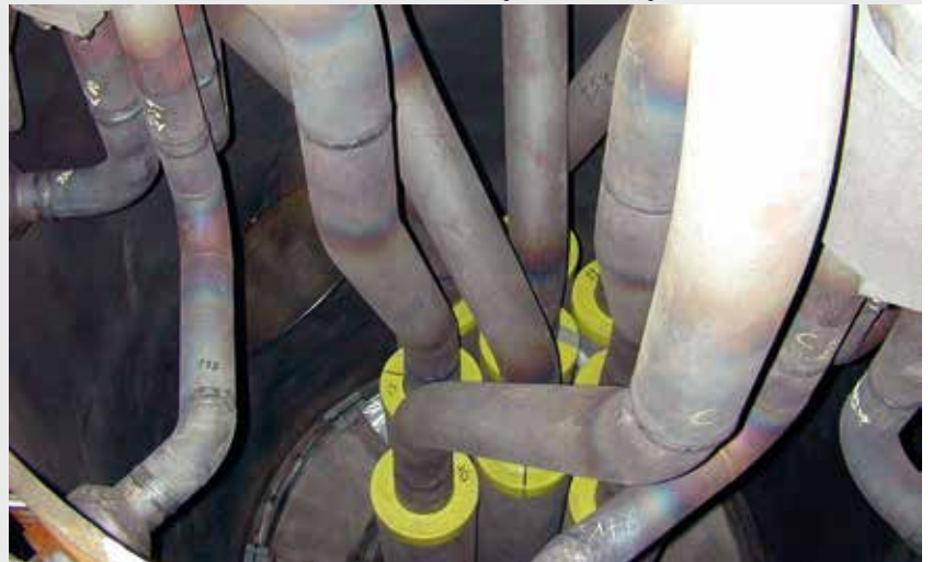
Assembled tubing between heating surfaces and inlet section
