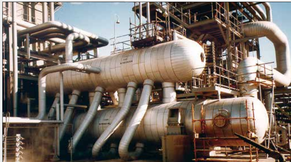
Process gas waste heat system
