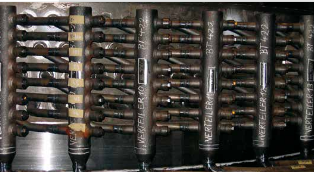
Inlet headers for LaMont waste heat boiler
