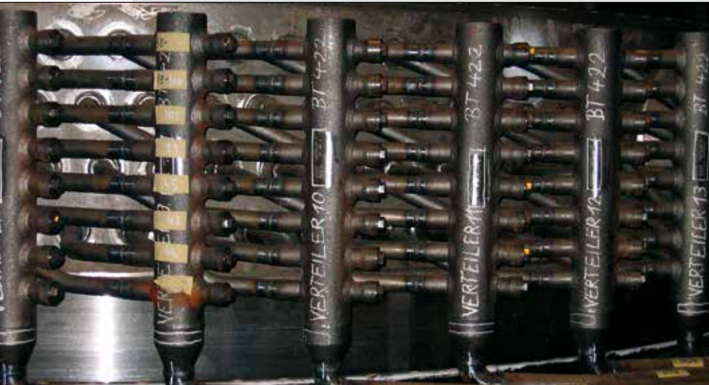
Inlet headers for LaMont waste heat boiler
