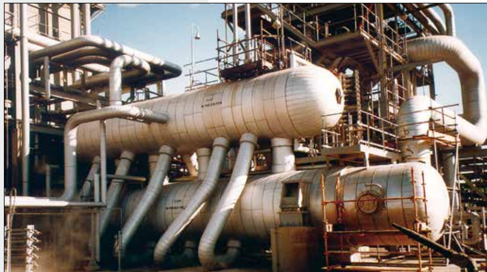
Process gas waste heat system
